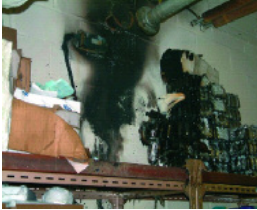
Figure 4: Fire in a storeroom (hot works) (courtesy of Network Rail)
